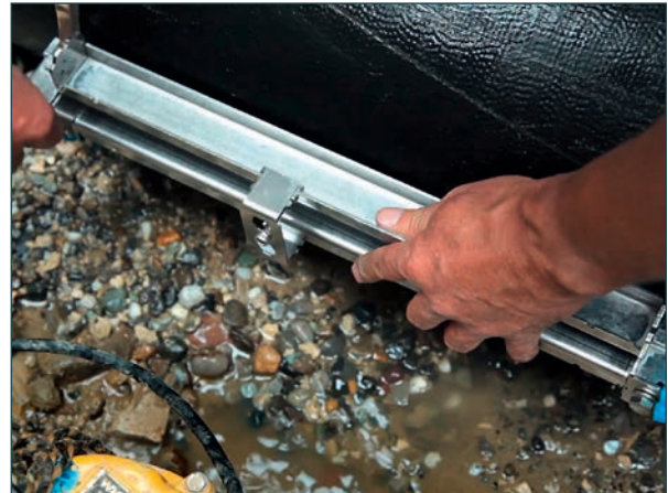
Fast installation without supply interruption
